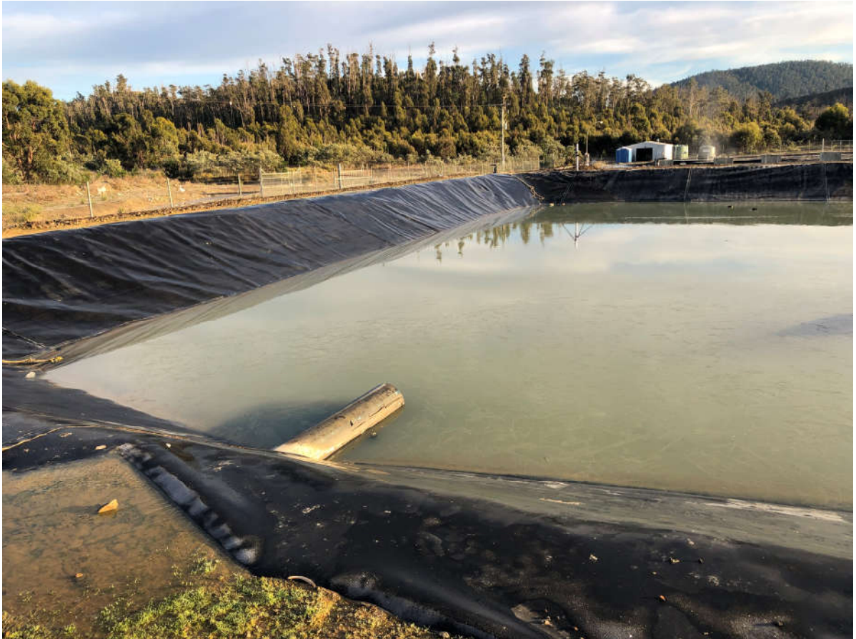
B-Cell Secondary Stormwater Pond (SS2)
