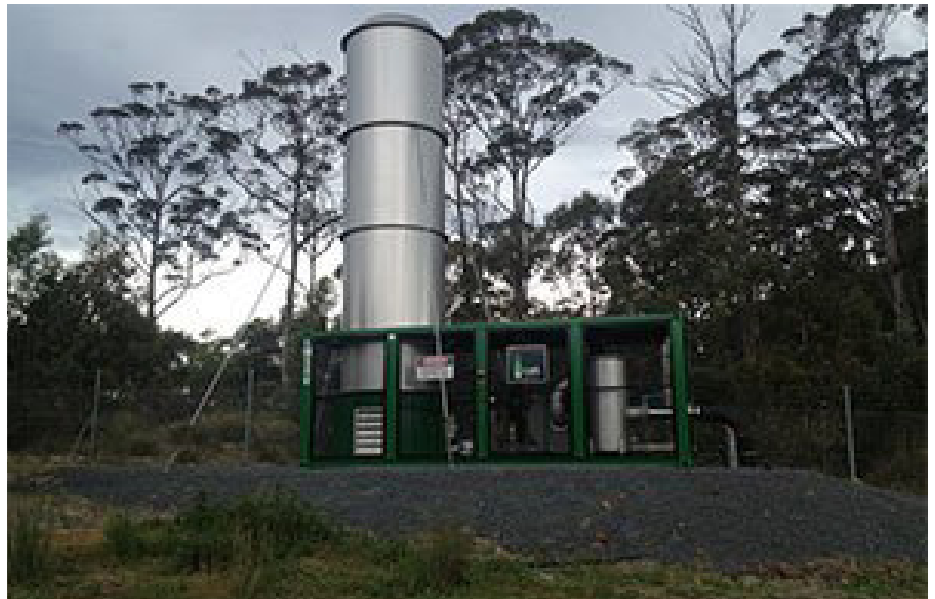
LMS Flaring Facility located at the Copping Landfill
